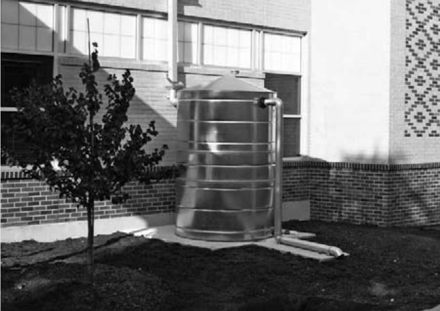
Langford Elementary Rain Collection Silo
